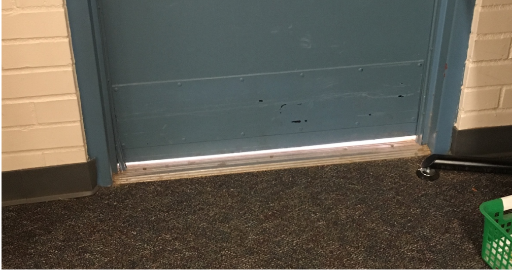
Figure 8. Light “leaks” around doorways are indicators of “open” doors for house mice. Photo: Shujuan Li, University of Arizona
