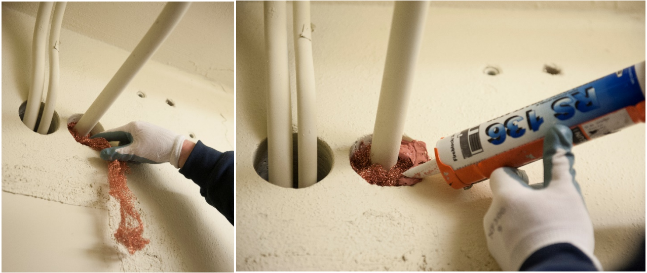
Figure 6. Sealing around conduits penetrating walls. Stuff gaps with Xcluder® cloth then seal with a siliconized acrylic latex or polyurethane sealant. Photos: Lynn Ketchum, Oregon State University
