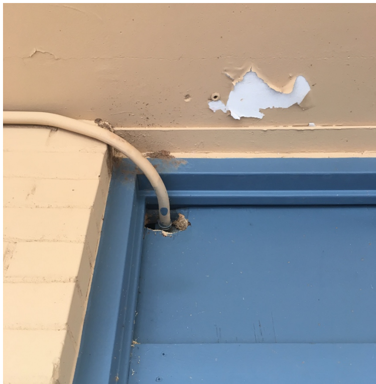
Figure 7. The gap around the wire passing through the door frame needs to be filled. Photo: Shujuan Li, University of Arizona
