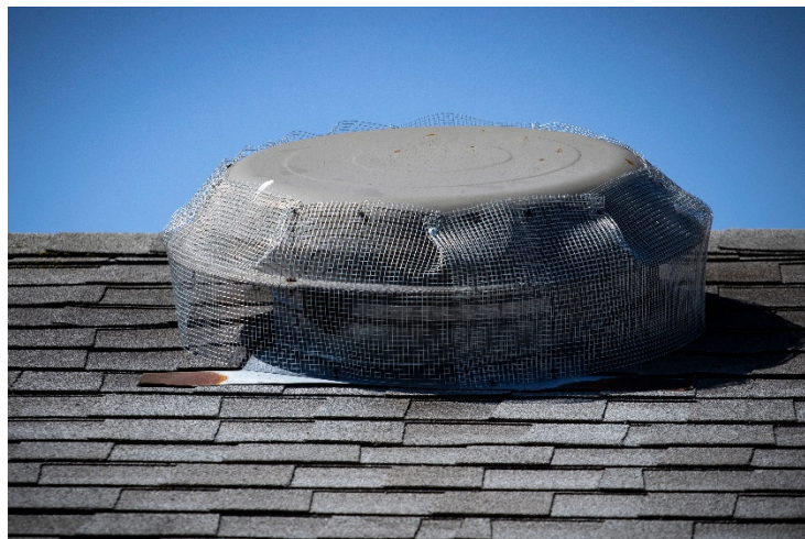
Figure 9. Exterior mesh on attic vents preventing entry of pests. Photo: Shutterstock
